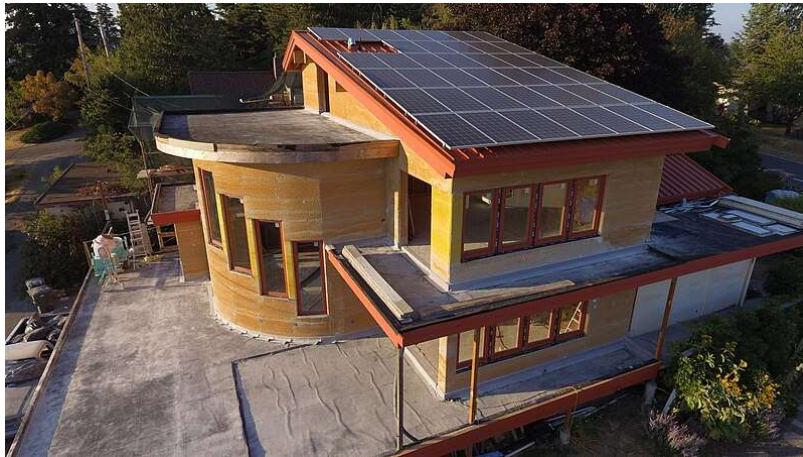
Figure 3: 3000+ square foot Highland Hemp House in Bellingham, Washington after the hempcrete is cast and before the plaster is added. (Tommy Gibbons, 2018)
